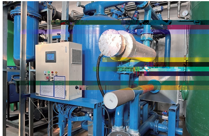
Zero Air Loss Blower Type Suction Dryer
