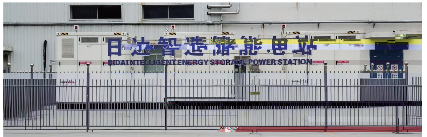
Energy Storage Power Station
